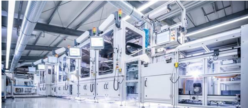
The automated production line handles dispensing, sealing, screwing, crimping and testing in a single plant. Video: https://youtu.be/E4sYP1J_UZQ
